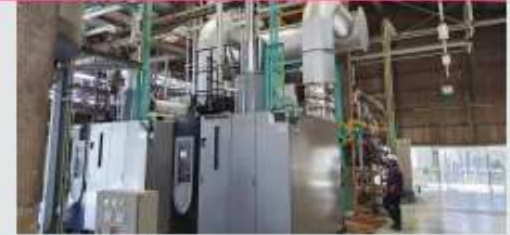
Boiler (Thailand) The Kansai Electric Power Co., Inc.
