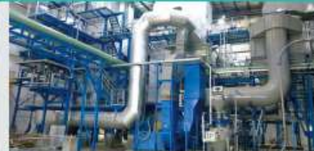
Biomass Boiler (Vietnam) Daichi Jitsugyo Co., Ltd.
