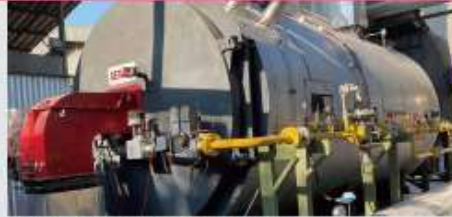
Thermal Oil Heater System (Indonesia) Fumakilla Limited
