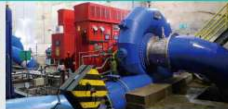
Mini Hydro Power Plant (Indonesia) Volth Fuji Hydro K.K.
