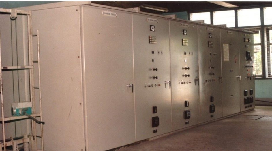
Control Panel Room Booster Pumping Station No.(1) 7/9/2018
