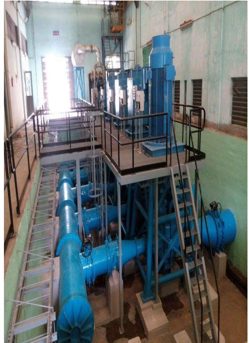
410KW Booster Pump – 4 units
