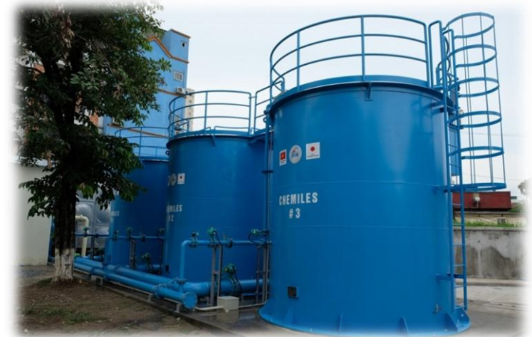
CHEMILES system in Hanoi Water Co. Ltd.
