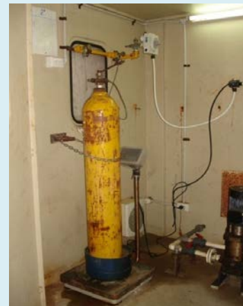
Chemical usage in SW treatment
