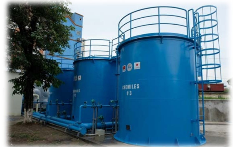
CHEMILES system in Hanoi Water Limited Company
