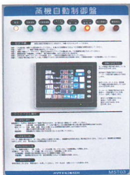
Steamer control panel
