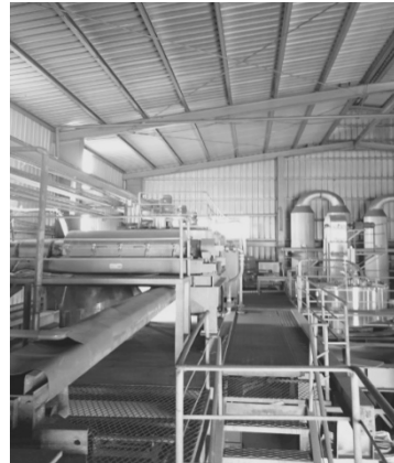
Slurry Plumbing System
