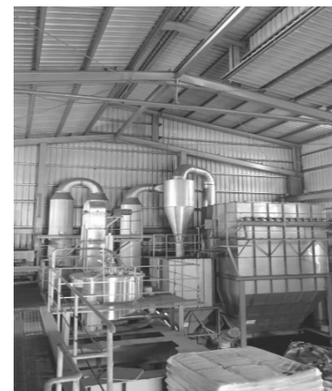
Dryer + Power Collector
