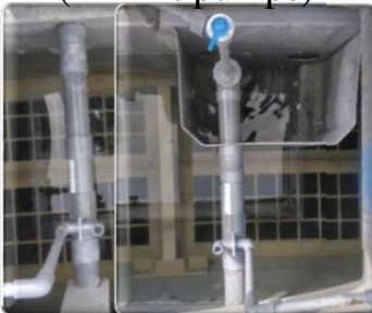
Adjust water transfer (Air lift pumps)
