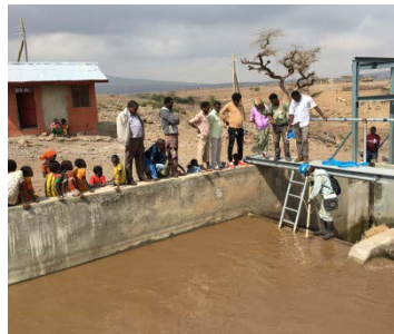
Community members observing works on the ULH-MHP system in Fentale (Ethiopia)
