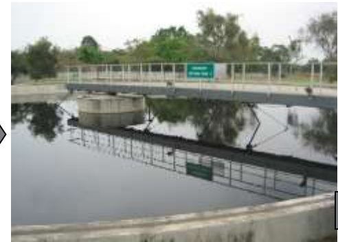
FINAL SEDEMENTATION TANK
