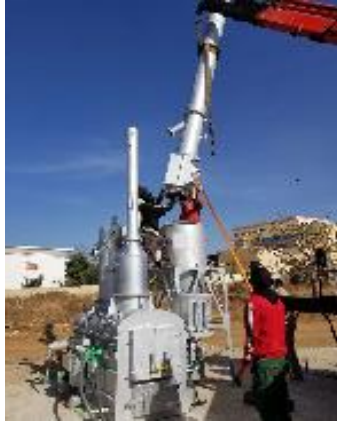
Senegal Incinerator installed in Senegal
