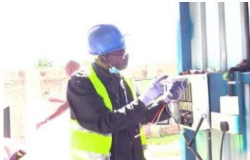
Kenya Installing and assembling an incinerator for medical wastes at the local site
