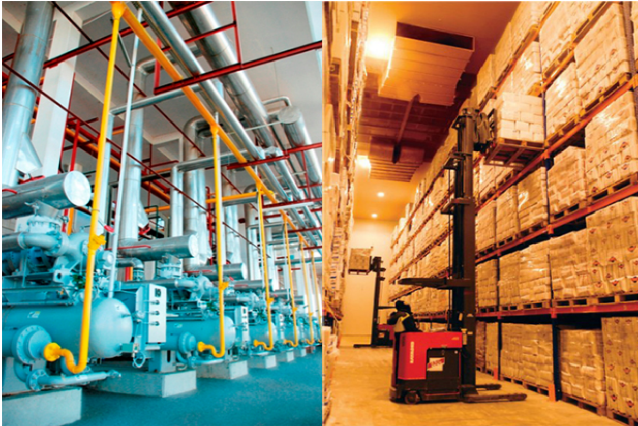
Screw compressors in the machine room
