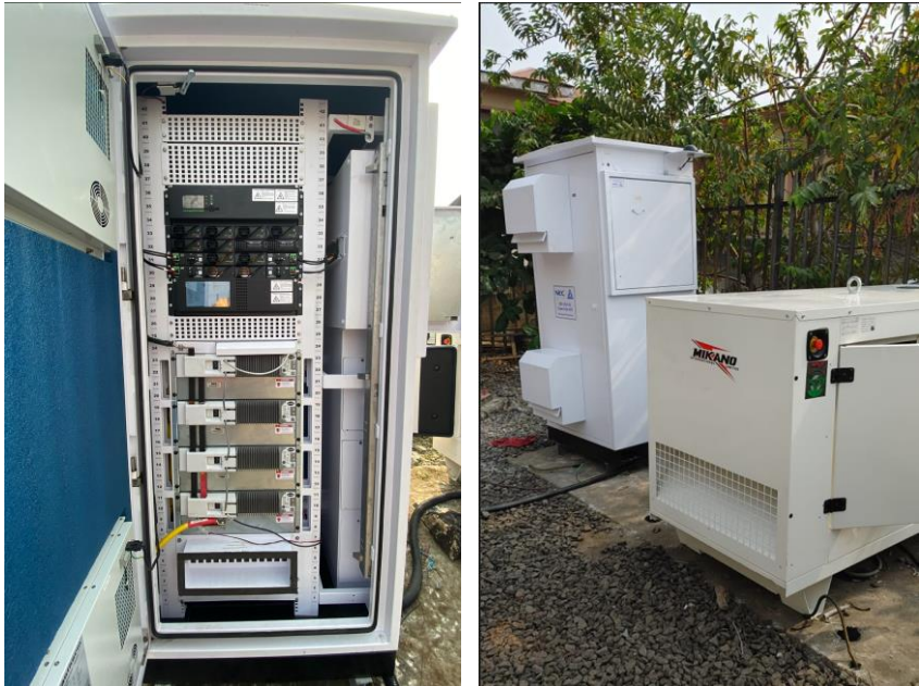
NEC Hybrid Energy Battery Storage
