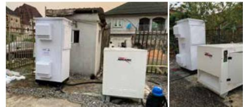
Our hybrid electricity storage system, which has been introduced to numerous countries
