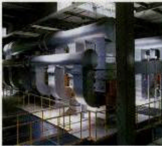
Flue gas treatment
