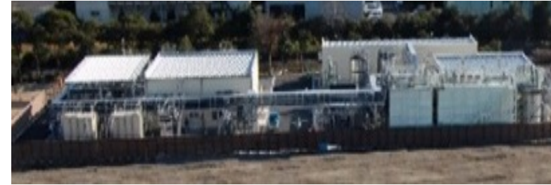
Verification Plant in Kitakyusyu (2011-2014)
