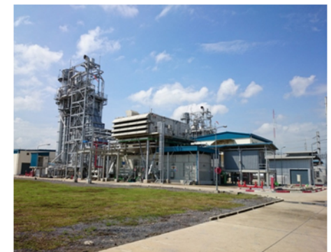
Gas power Projects in Matola and Temane(EPC:Sumitomo)
